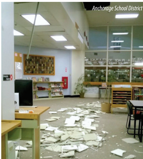
The 2016 M7.1 Iniskin Earthquake damaged ductwork and ceiling tiles at Romig Middle School in Anchorage.
